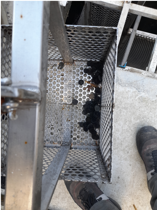
Figure 9 Basket installed just before discharge allowing biocarriers collection ©AcquaPublica
