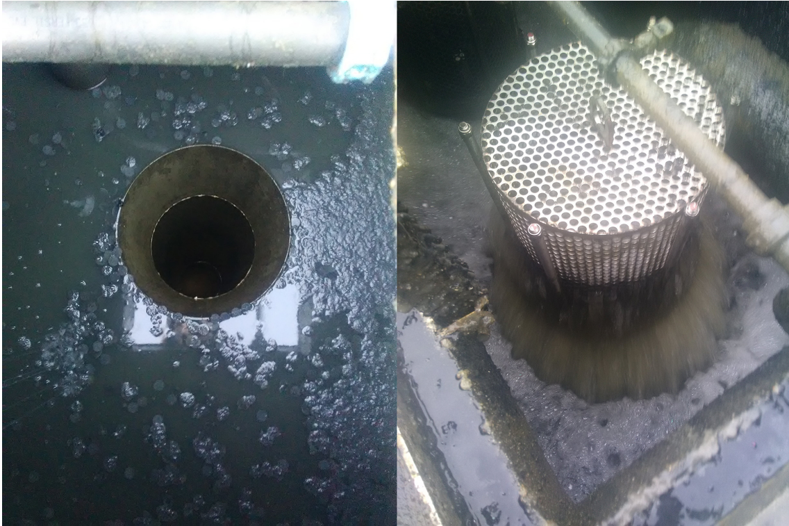
Figure 7 Installation of a strainer (right) on a discharge opening in a biological treatment tank, 2020 ©AcquaPublica
