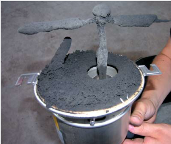
Figure 10: Electrode clamp of the Zumikron ESP, demounted for cleaning
